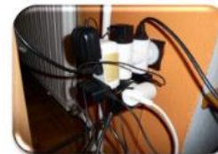
Do not overload power outlets
